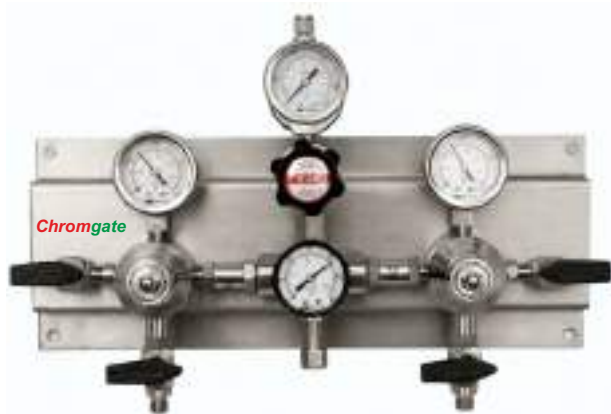
AUTO CYLINDER CHANGEOVER PANEL
